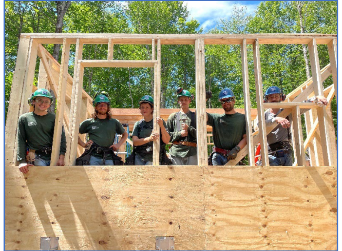
VYCC's new "Pro Build" crew is building a 4-season hut in the Green Mountain National Forest. Once footers are installed, they are responsible for all construction, from the floor joists up to the roof.
