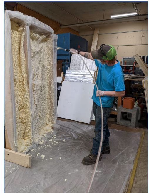
A Serve Learn & Earn participant in a ReSOURCE Weatherization 101 course sprays high-efficiency insulation.
